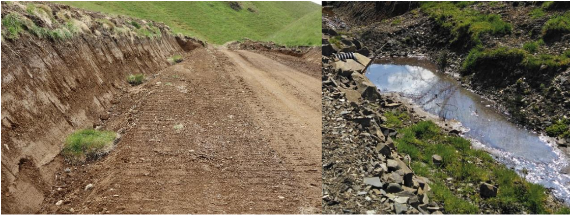
Above – Left – Example turf bunds on new formation. Right – Silt trap installed before culvert.
