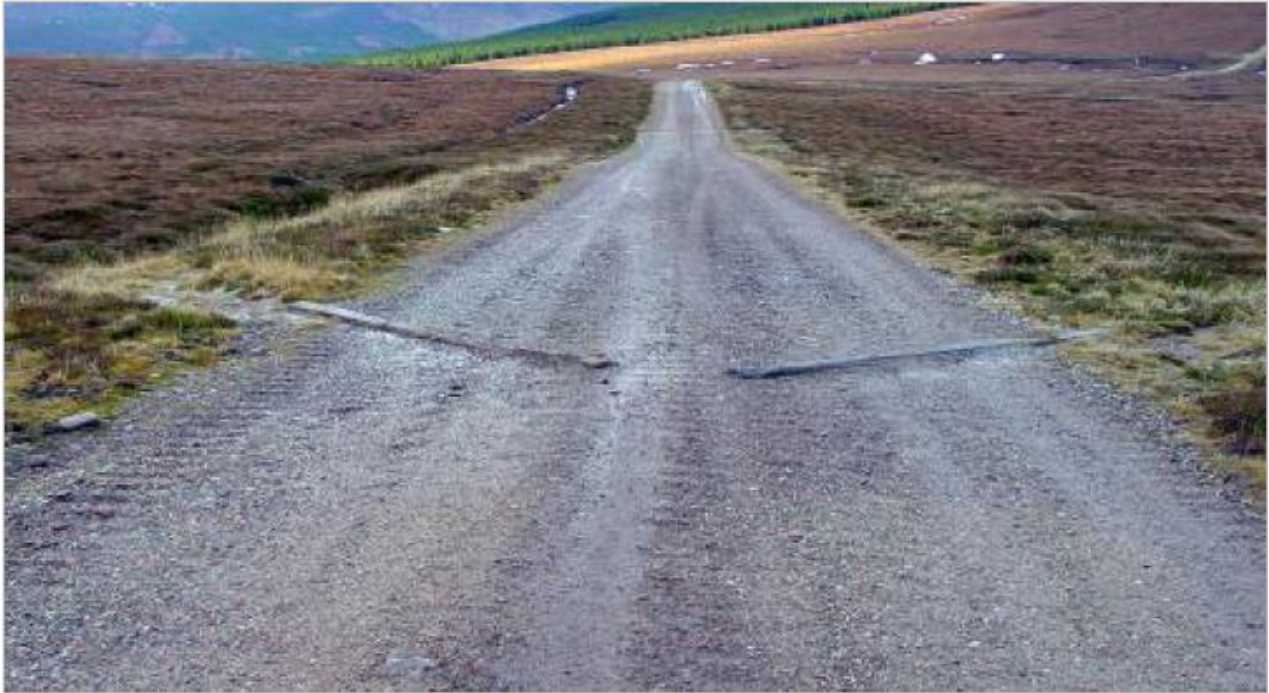
Above – example cross bars set in road to shed water in both directions.
